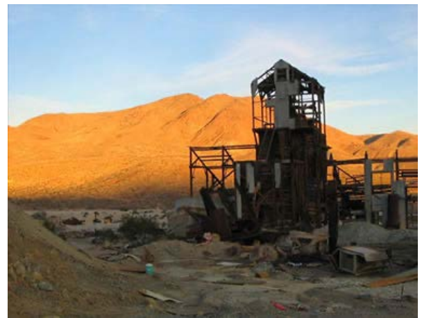
Abandoned mine structure: Structures at abandoned mine sites are often dangerous and unstable. They can also house dangerous chemicals or explosives. Stay out of these structures. Bureau of Land Management image.
